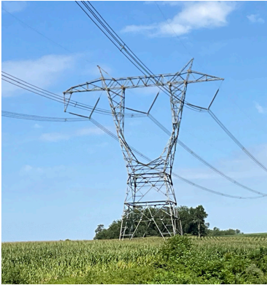
Typical 765-kV transmission line structure
