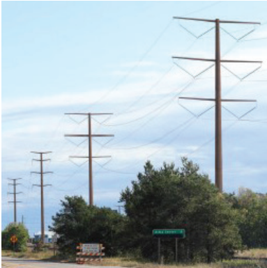
69kV double-circuit structure
