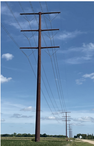
Example of double-circuit 345-kV structure.
