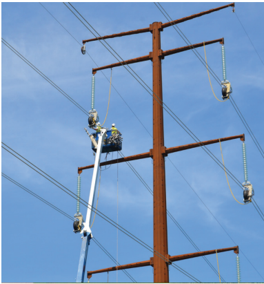
Typical 345-kV transmission line structure
